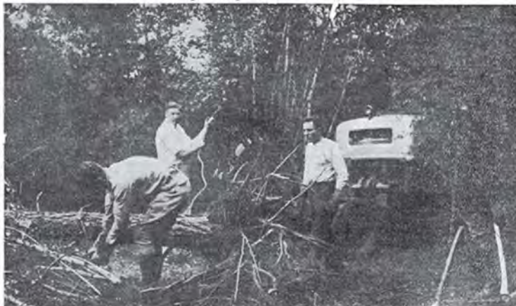
Above shows action in clearing land for the Saratoga County Central Airport on the Milton Plateau south of Ballston Spa and South of Saratoga Springs. One runway is about completely cleared. Workers hope to have the 'port' cleared for planes this fall. Photo shows Bryan Morley releasing cable from tree just pulled out, with Harold Cull letting up tension on the winch. Robert Shortleaves, truck and winch operator, is walking up to help Morley. Postmaster Edward J. Morley stands behind trees in the foreground.
